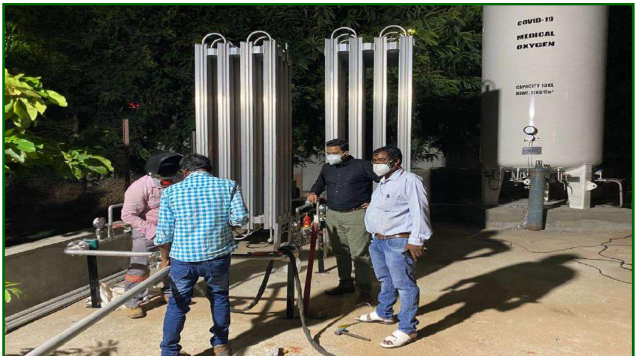
Extended assistance for converting Samras Hostel, Vadodara into Samras COVID care Hospital including fabrication of SS piping for the supply of Vaporized Oxygen and assembling of Ventilators.
